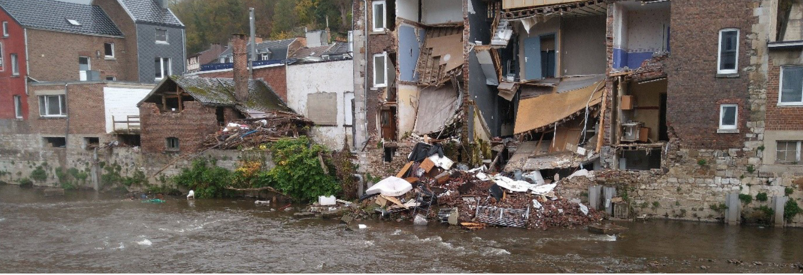
Residential building with significant structural damage in Pepinster, Belgium, located at the bank of the Vesdre River, upstream of the confluence with the Hoegne River. (Source: RMS, November 2, 2021)
