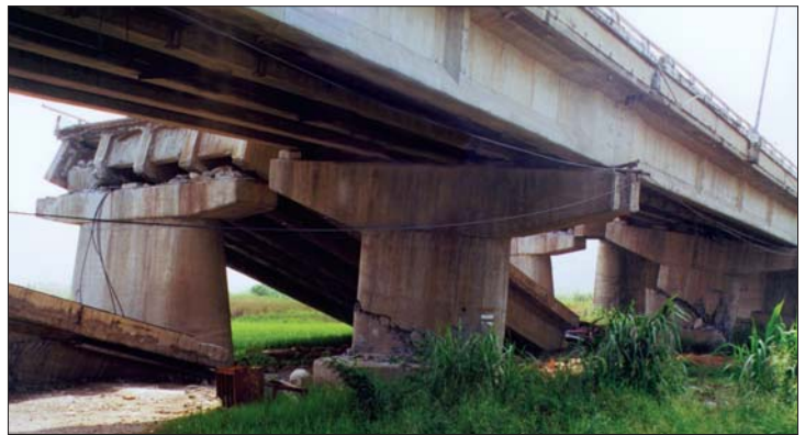
On Tai-3 near Wufeng, the Chelungpu Fault rupture sheared through a bridge column, causing several spans to collapse.
