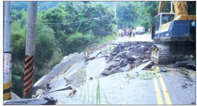
Landslides caused most of the more than 600 road disruptions, limiting access to remote mountain villages for more than a week and hampering emergency operations throughout the epicentral region.
