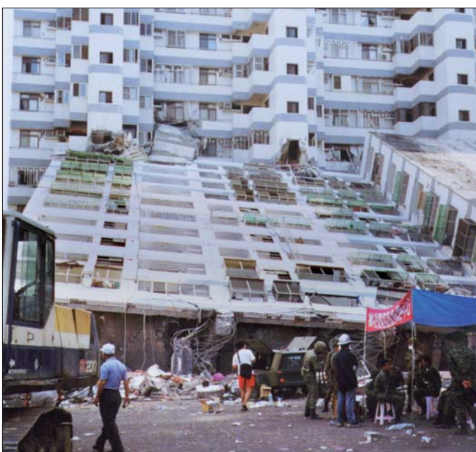
The combined vertical weight of the building and earthquake overturning forces exceeded the load-bearing capacity of the columns, completely toppling some buildings, such as this one in Dali.
