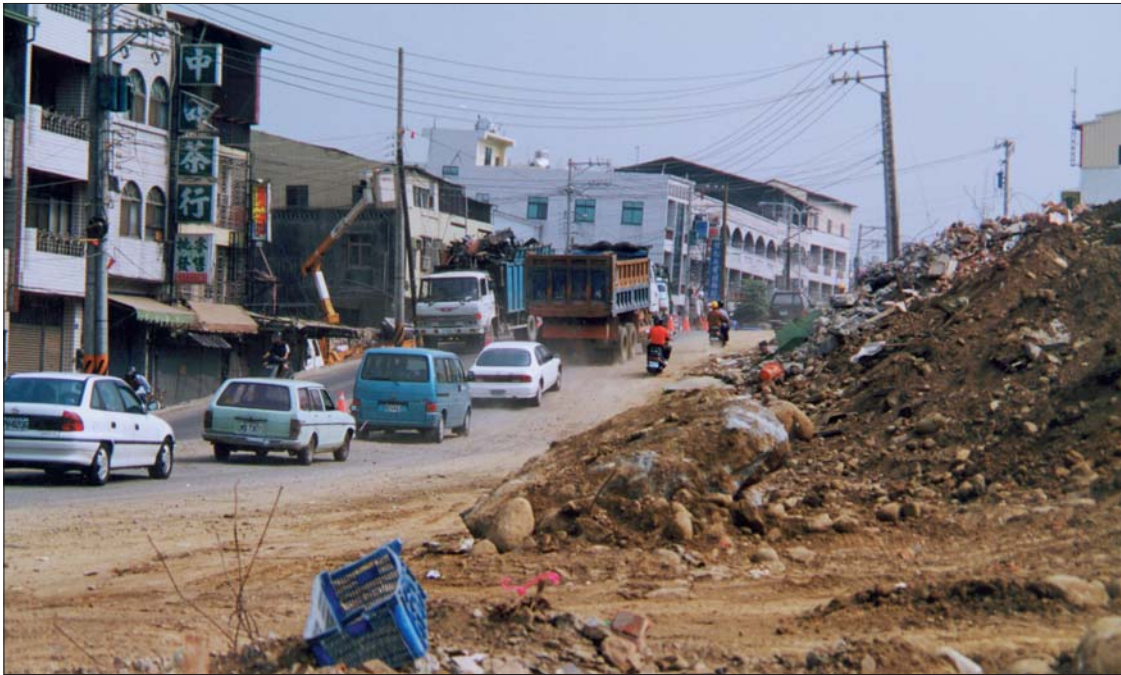
The Chelungpu Fault rupture and associated warping damaged buildings, infrastructure, and roads in Fengyuan. New maps have been prepared with construction setbacks from fault lines (similar to California's Alquist-Priolo zone requirements).
