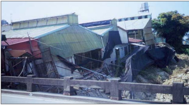
Ground deformation associated with the earthquake faulting destroyed these lightweight structures and formed a dam across the riverbed near Fengyuan.
