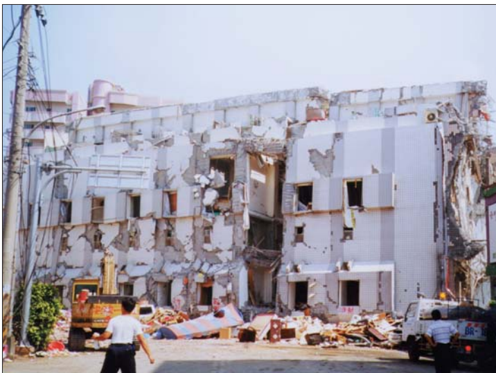
A completely overturned high-rise apartment building in Dali. Taiwan will have to come to terms with apparent code and construction practice deficiencies in the months ahead.
