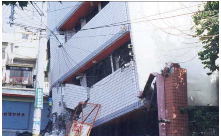
The non-ductile concrete frames in many buildings' first floors collapsed when they were unable to withstand the lateral earthquake forces.
