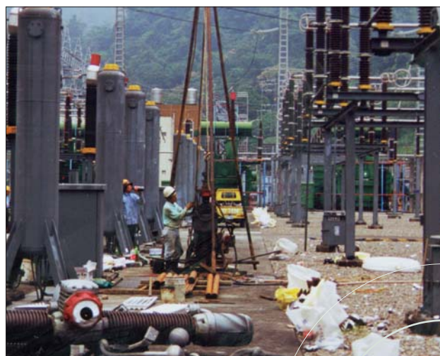
Clean-up underway at the Tienlun switchyard, nearly one month after the earthquake. Similar heavy damage that occurred at the Chungliiao substation was already cleaned up by this time.
