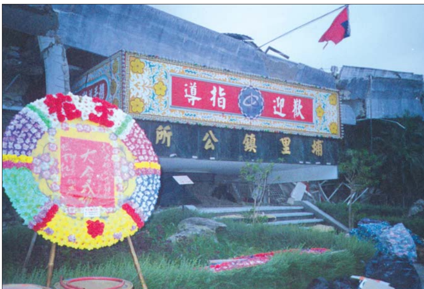
The 4-story reinforced concrete city administration building in Puli also suffered a pancake collapse.
