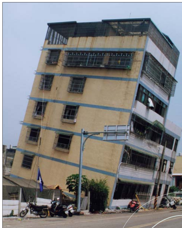
A partially collapsed reinforced concrete building in Dungshr. Approximately 15,000 buildings were heavily damaged or destroyed, the majority of which were mid-rise reinforced concrete structures.
