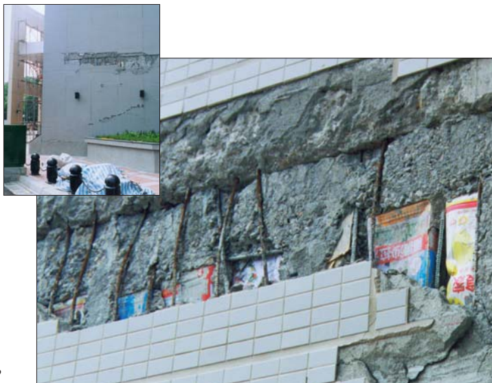
Spalling on the exterior veneer exposed salad oil cans in the concrete beams of this newly constructed reinforced concrete building in Nantou City.
