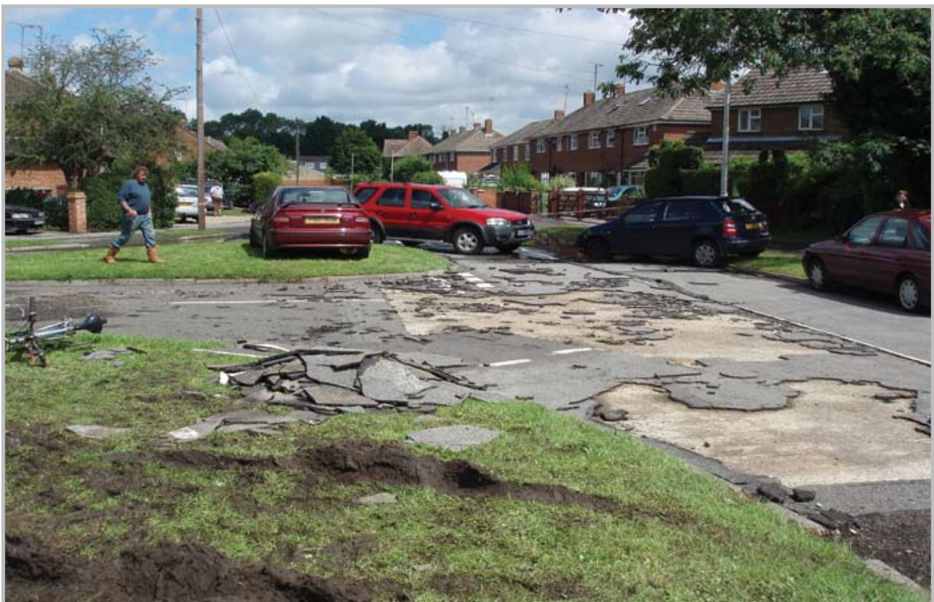
Figure 7: Roads were badly damaged during floods
